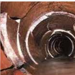
POTENTIAL POOR PIPES AND SERVICES
