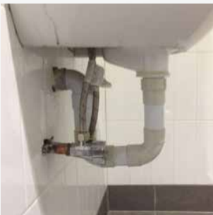
POOR PLUMBING MARK OUT
